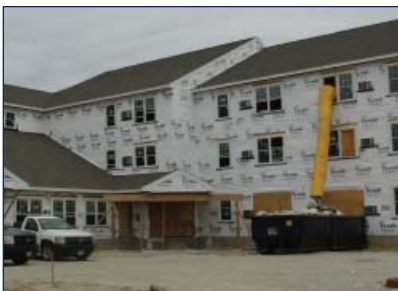
South Porter Street: Manchester, NH Sponsor: Manchester Housing & Redevelopment Authority Units: 31 senior Architect: Dennis Mires, PA Permanent lender: New Hampshire Housing Construction lender: New Hampshire Housing General contractor: Fulcrum Associates Construction jobs saved or created: 34
